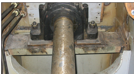
Figures 37: Poor construction of shaft line foundations.
