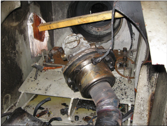
Figure 40: Fatal damage due to resonance problems.
