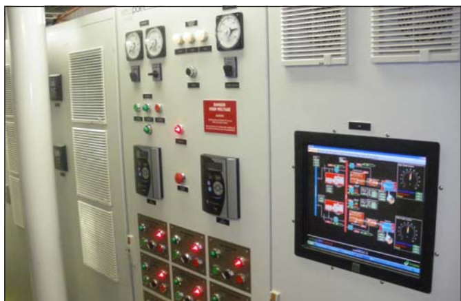
Figure 5: Main switchboard/hybrid control system showing engine room console.
