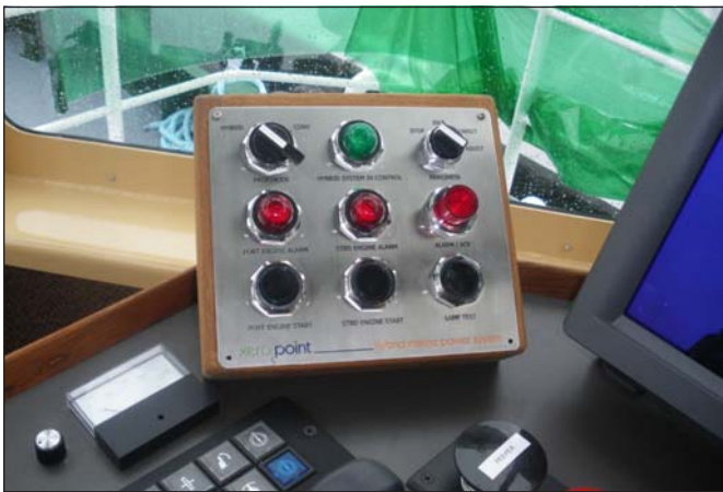
Figure 7: Hybrid system control panel.
