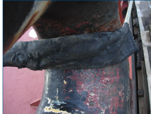
Rough finish as coating wears away.
