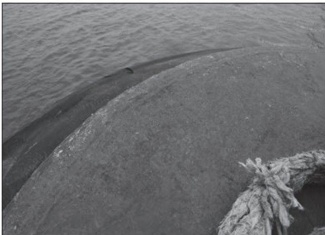
Figures 3a & b: Bull nose contact surfaces; rough surfaces causing heavy surface abrasion.
